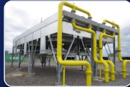
Ambient Heat Exchangers
